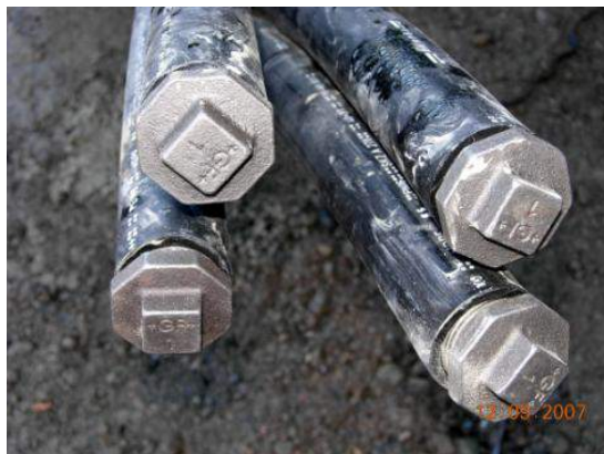
Figure 8. Example for sealing the BHE after final testing (picture: Polydynamics Engineering Zurich)
