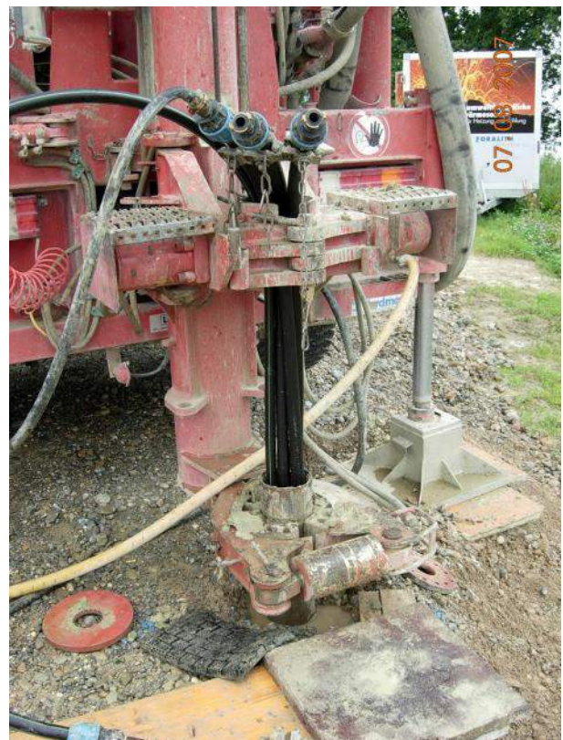
Figure 7. During grouting the auxiliary casing still prevents the borehole from collapsing. The BHE is under pressure (picture: Polydynamics Engineering Zurich)
