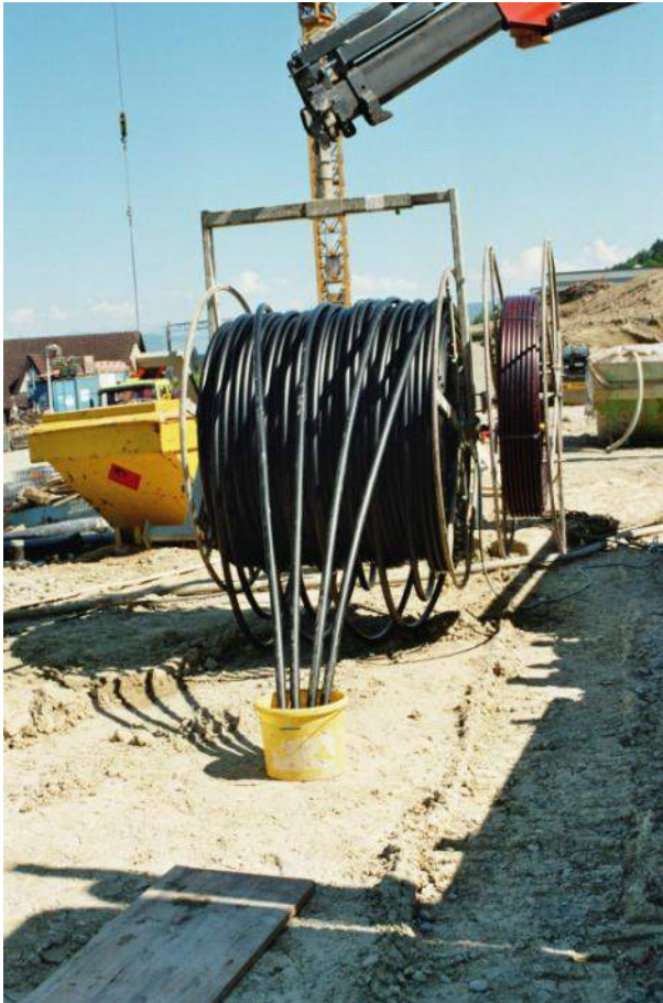
Figure 1. BHE on a decoiler during the first density test using air (picture: Polydynamics Engineering Zurich)
